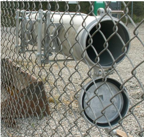
Storage canister for hot stick attachments attached to station fence in all stations.
