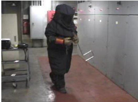
Arc flash suit to be used when operating or racking metal clad type switchgear.
