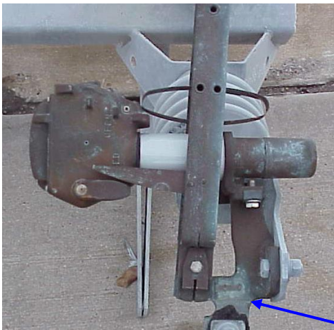
Figure 4 Partially closed switch. Note that the contact bayonet and the contact jaws are only partially engaged.
